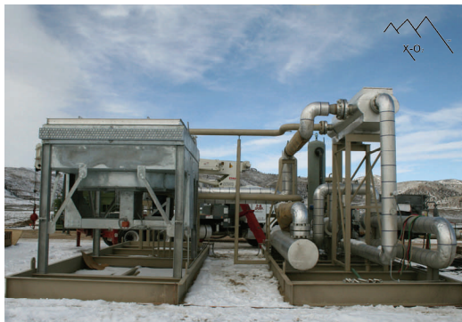
10 MMSCFD Oxygen Removal Plant
